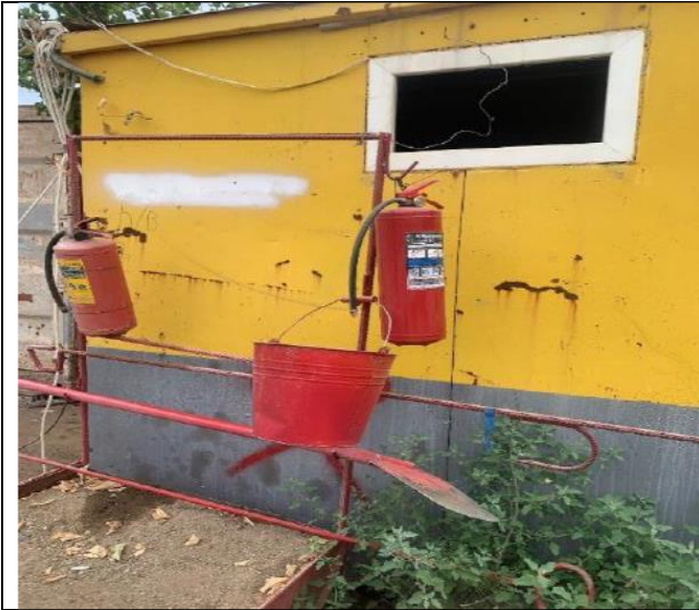
Fig -9 -Camp is equipped with firefighting equipment. 13.08.2025
